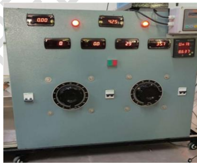
Figure 3: An electrical panel
